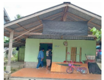
A house in Ujung Baru 1 Village, East Luwu, built with 50 cm concrete blocks and planks above them.
